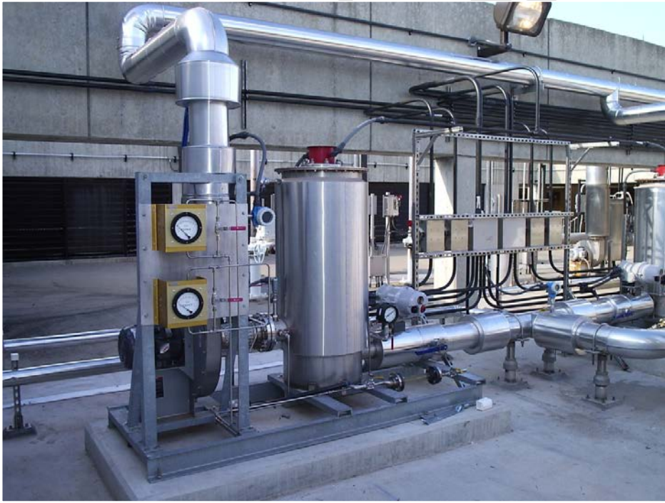
Figure 6-7 Ozone Offgas Blower and Destruct Unit Skid at Fairfax Water Corbalis WTP
