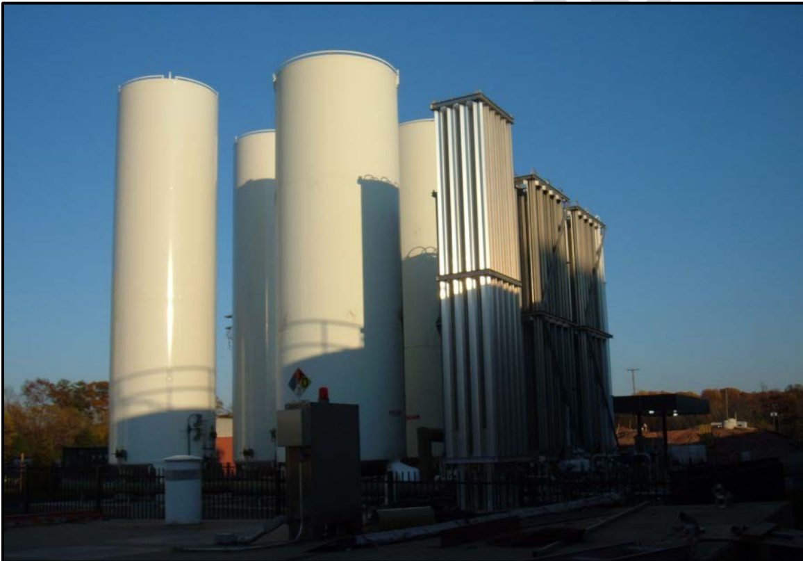
Figure 6-4 Vertical LOX Tanks and Ambient Air Vaporizers at Corbalis WTP
