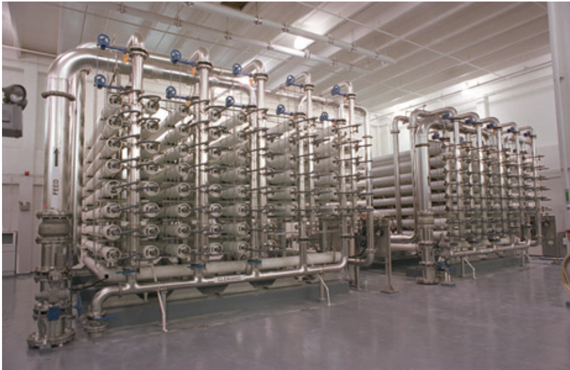
Figure 5-5 Two-Stage RO Membrane Skids Using Standard 8-Inch Diameter Pressure Vessels
