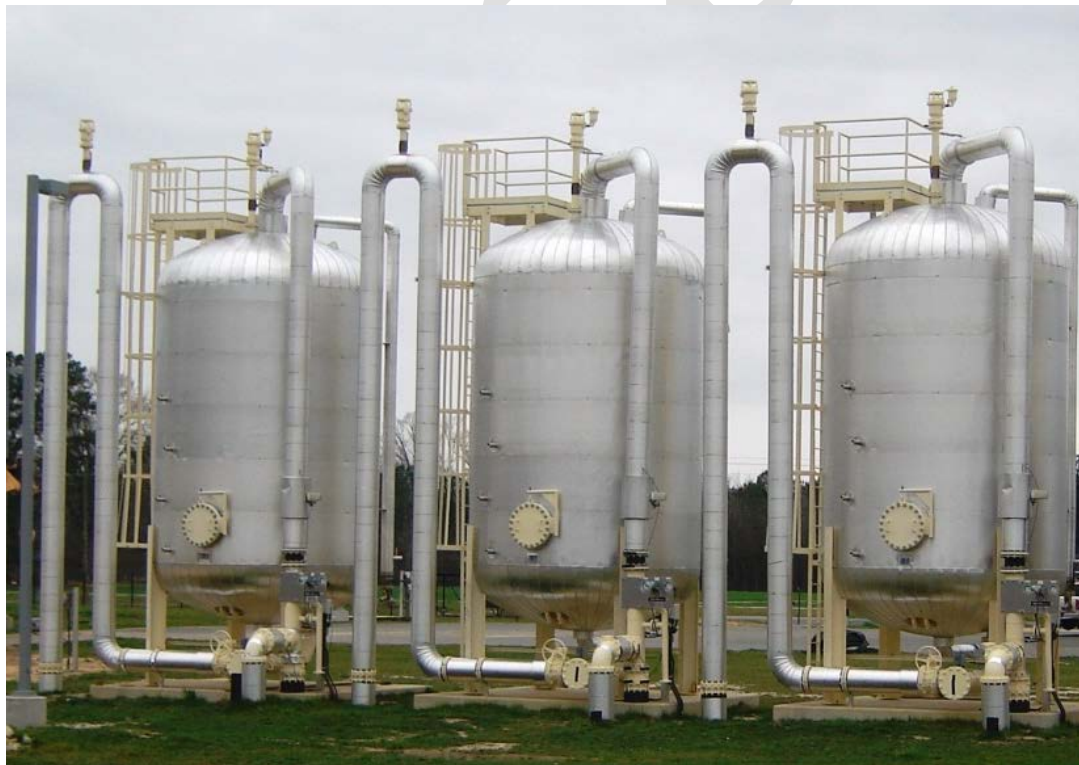
Figure 3-3 GAC Pressure Contactors
