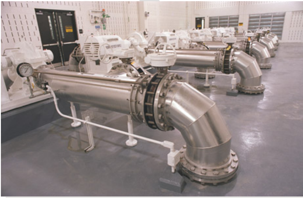
Figure 5-4 Horizontal Split Case RO Feed Pumps
