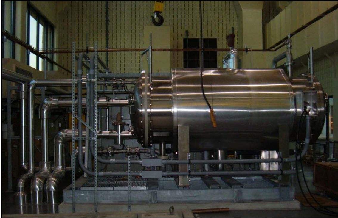
Figure 6-5 Ozone Generators at Corbalis WTP
