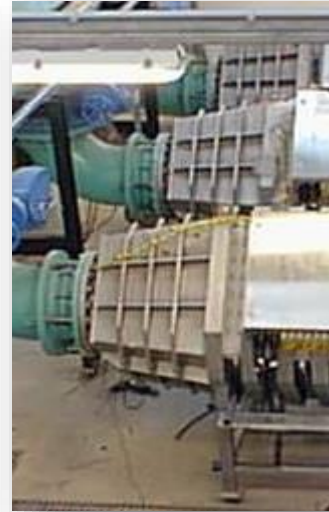
UV-Advanced Oxidation Process (UV-AOP)
