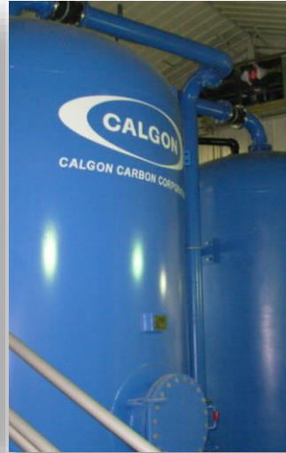
Granular Activated Carbon (GAC)
